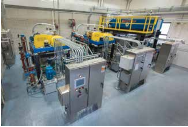
The centrifuge room at the Kenosha Water Utility
